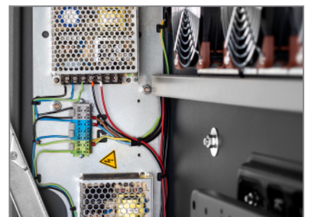
Cabling according to VDE guidelines
